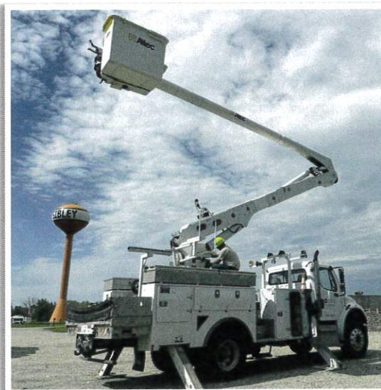
Louie proves he can use the lower controls to safely lower the bucket to the ground.
